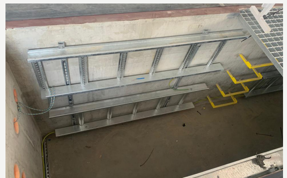
Cable Ladder in Cable Pit
