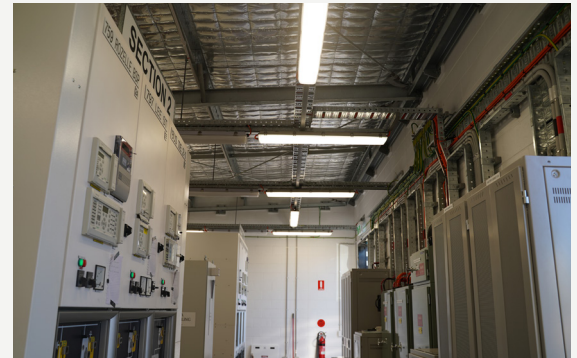
Switchgear Battery Charger Cabinets and Internal lighting
