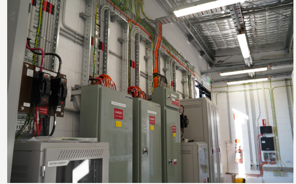
AC and DC Boards and Battery Chargers
